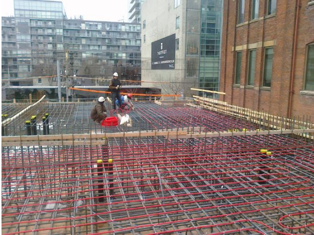
CIMG0141 REHAU PEXa pipes in rebar prior to concrete pour in commercial high-rise radiant heating/cooling system ©REHAU
