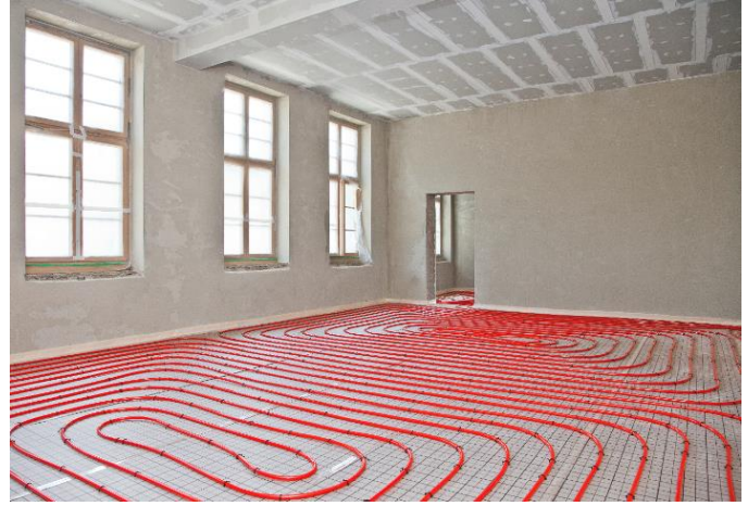
962-D023 REHAU PEXa pipes prepared for concrete overpour in radiant heating/cooling system ©REHAU
